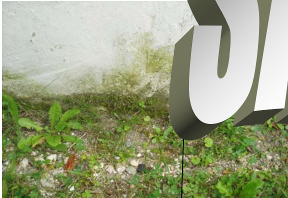
Mold and Mildew on stucco
