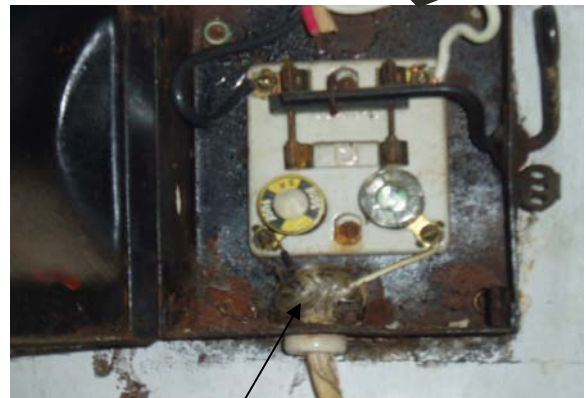
Loose BX sheathing
