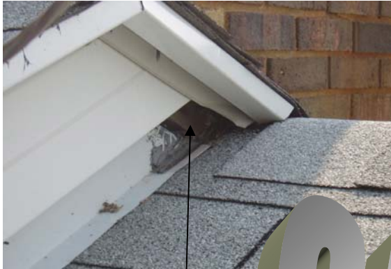
Missing piece of siding
