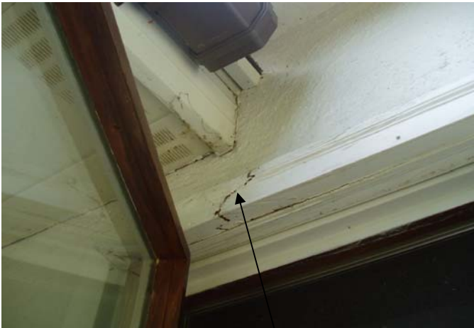
Wet rot above kitchen window
